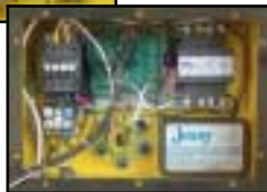
Electrical Junction Box
